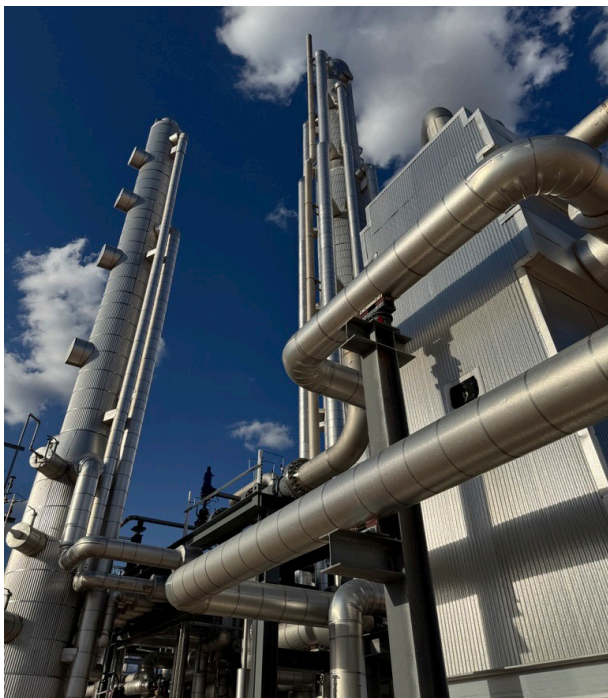
Figure 3. 125 million ft 3 /d NiTech IV two-column cryogenic NRU in New Mexico, US.
