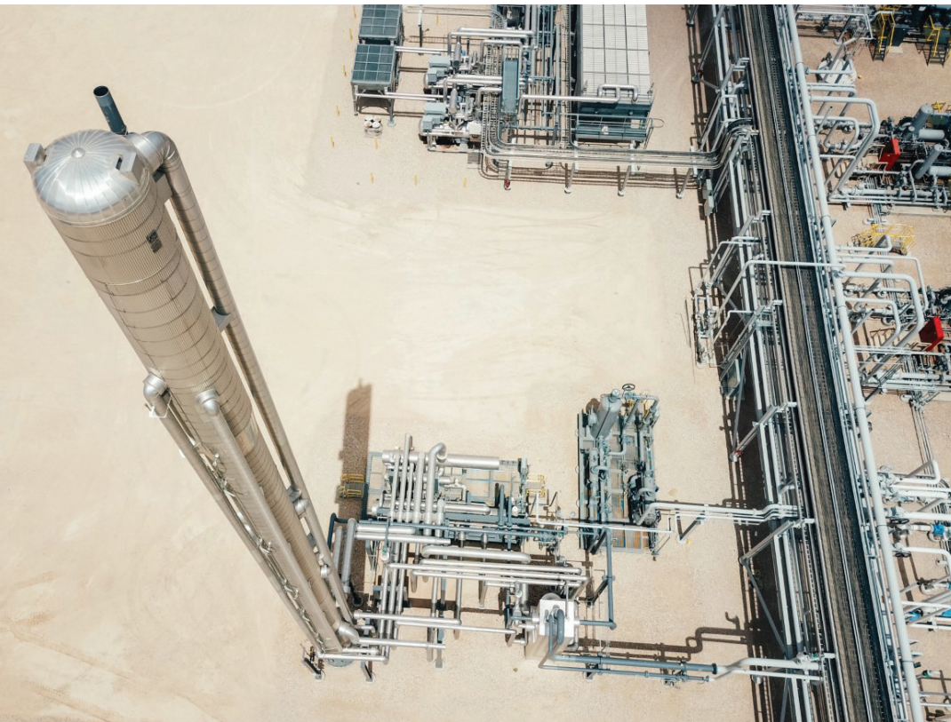
An Aerial View Of A NiTech Style III Nitrogen Rejection Unit (NRU)
