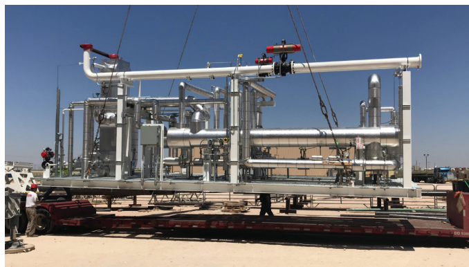
A NiTech Processing Skid
